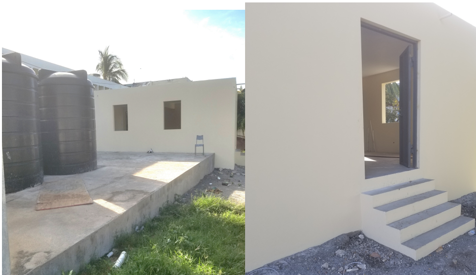
Housing for the pumps & purification plant and platform for 30,000 gallon tank.
