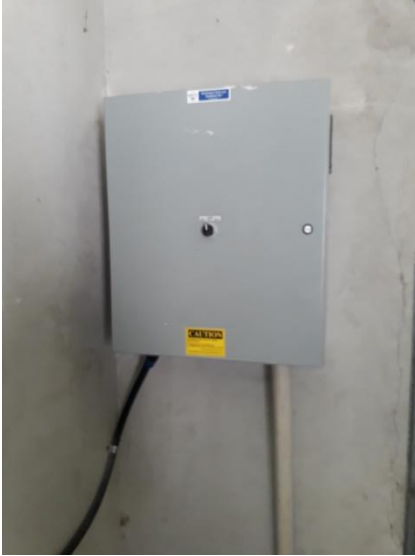
Fig 1 – VFD – Control Panel
