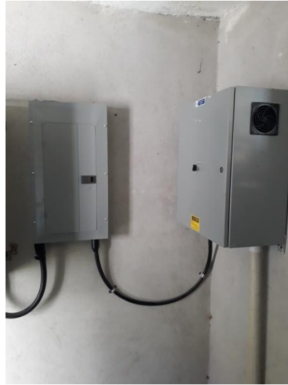
Fig 2 – Breaker Panel & VFD Control Panel
